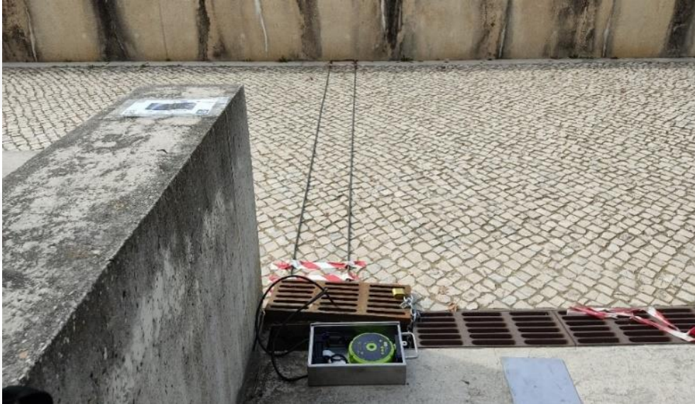
Figure 8 - Pneumatic tubes, which allows the detection of the passage of bicycles and e- scooters, installed at Access 2
