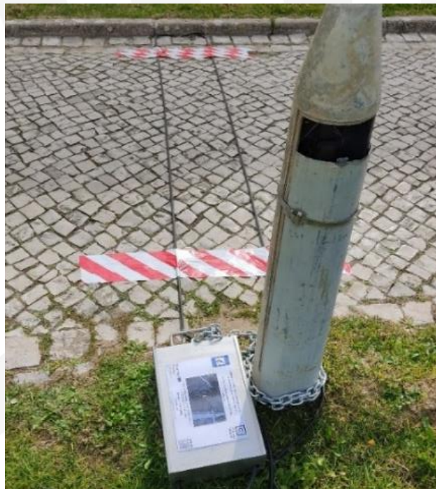
Figure 9 - Pneumatic tubes, which allows the detection of the passage of bicycles and e- scooters, installed at Access 3
