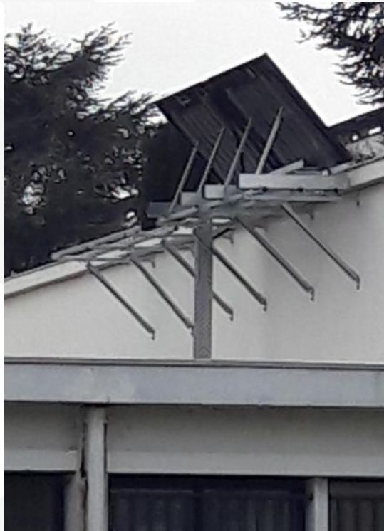
Figure 10. Dualsun solar panels mounted on the top of the building
