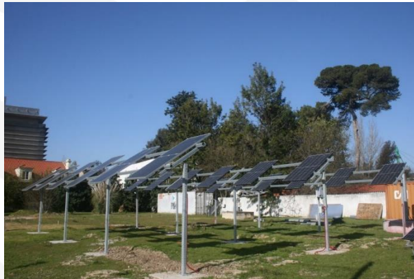
Figure 1. Outdoor PV system
