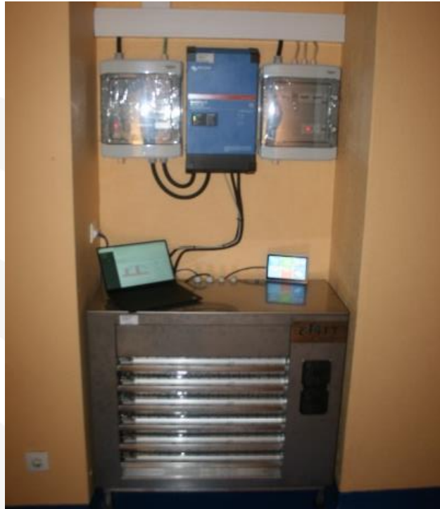
Figure 2. Indoor battery and control system
